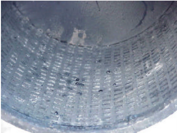
Safety filter of the blower
