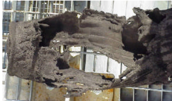
Damaged bag filter
